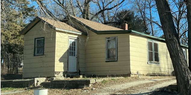
▲ Figure B.4: Single-Family Home Needing Moderate Rehabilitation
